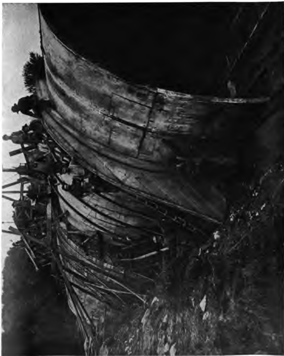
PLATE 144.—Contract 2. Cut-and-cover Aqueduct. First steel forms—McNally—used on Catskill Aqueduct. Outside forms are of steel ribs and wooden lagging. Wooden bulkhead contains steel plate to act as water stop at expansion joint.
